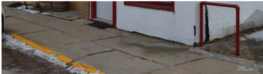
Figure 29. Uneven sidewalks pose tripping hazards for those with reduced mobility
