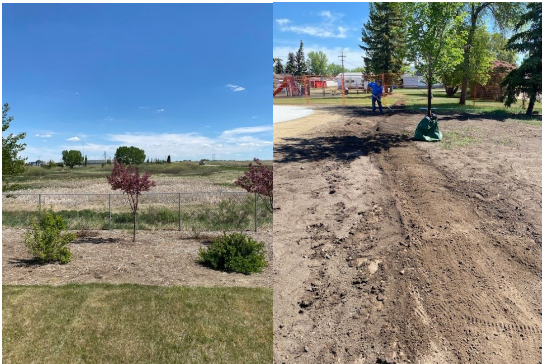
Tree replacement at VIC (left) and irrigation work at RCMP Park by Spray Park (right)
